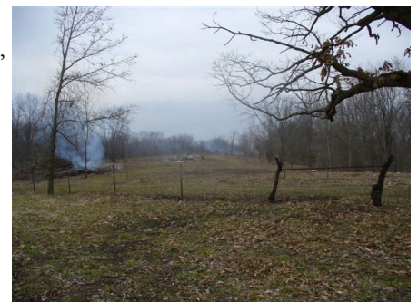
Brush piles still smoldering after invasive vegetation had been cleared from the site.
